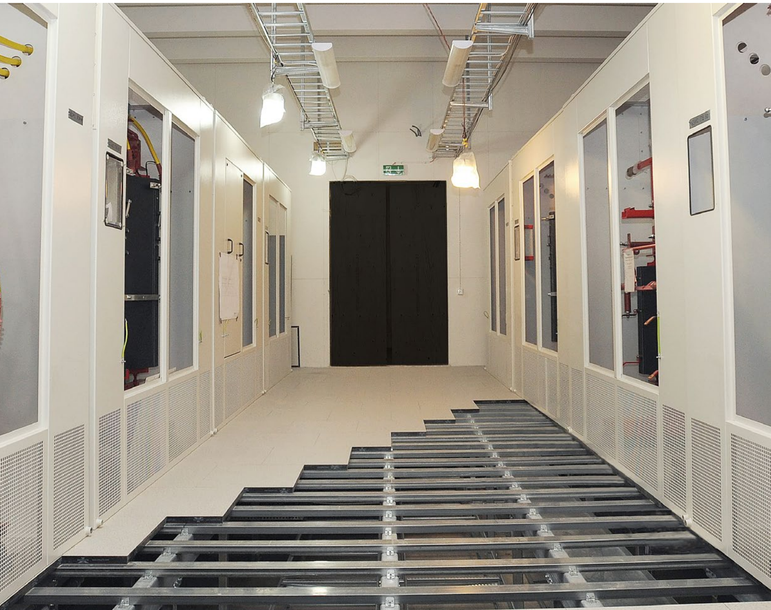
Transformer Room at Karolinska Hospital with reinforced Iso Floor Substructure supporting 16 Transformers with a total weight of 120 ton.
